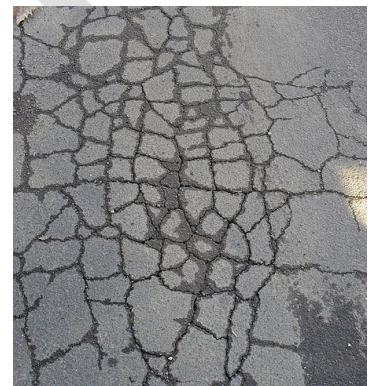
Figure 5: Section of asphalt showing alligator cracking, indicating poor surface condition in need of repair.
